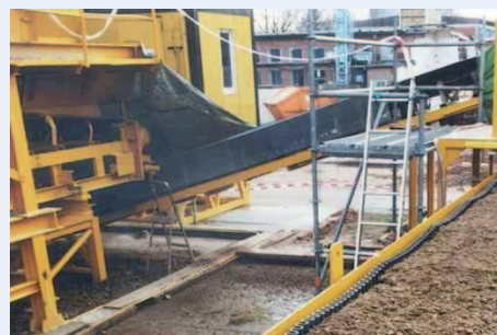
Release Measurement System for Loose Waste, NUKEM Hanau (GER)
